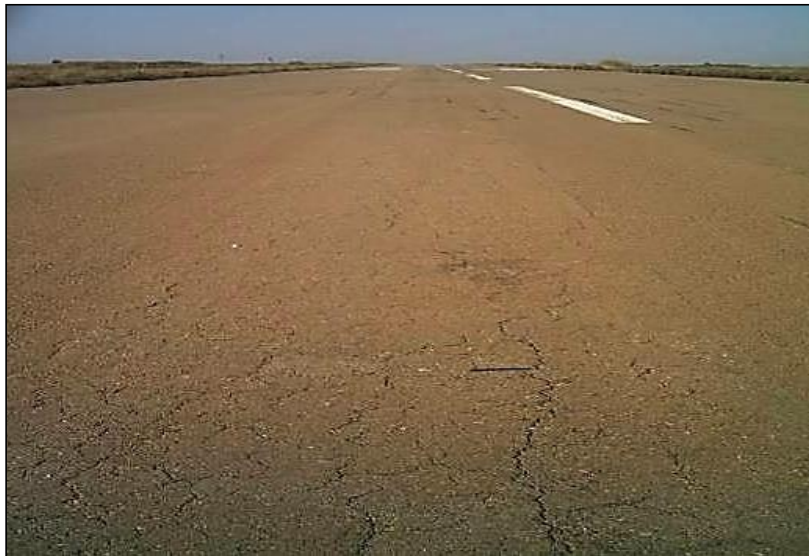
Fig. 2. Longitudinal cracking on the runway.
